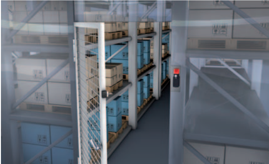
Economical solution: L10 Safety Locking Device on a door to the store area without control signal for the guard interlocking (manual locking and unlocking)
