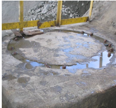
Damaged concrete base
